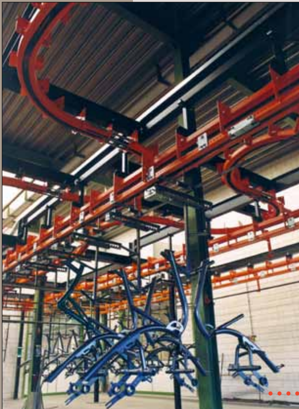
Power & Free conveyor .....
